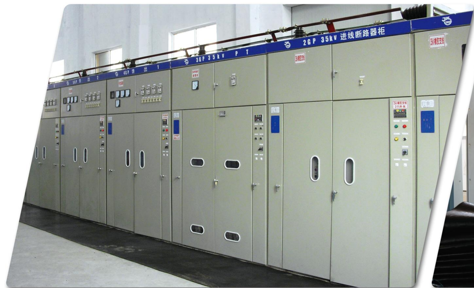
35KV变电站 35KV converting station
